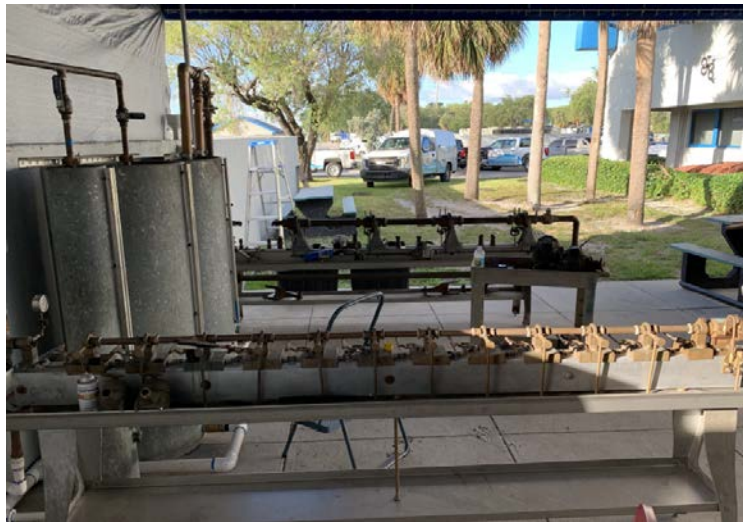
Exhibit 4.14 – Meter Testing Bay
