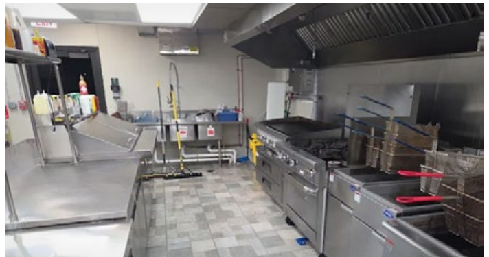
Commercial Kitchen at Provident Market
