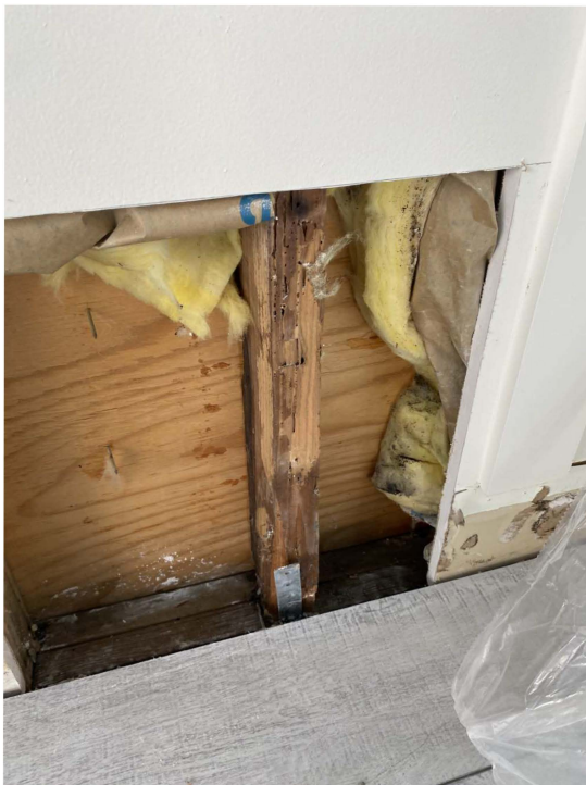
Photo 5: West Living Room Wall Stud
