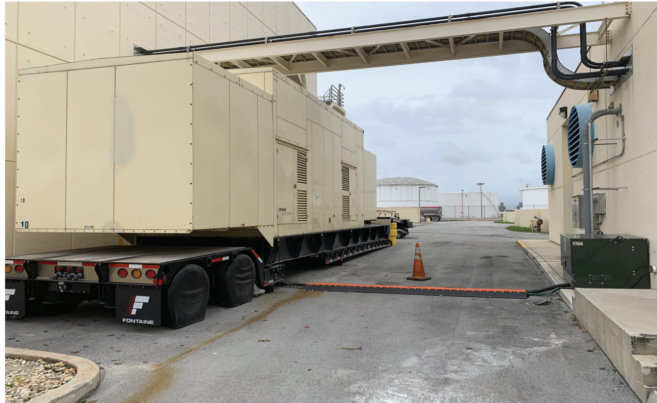
GTL Temporary Generator
