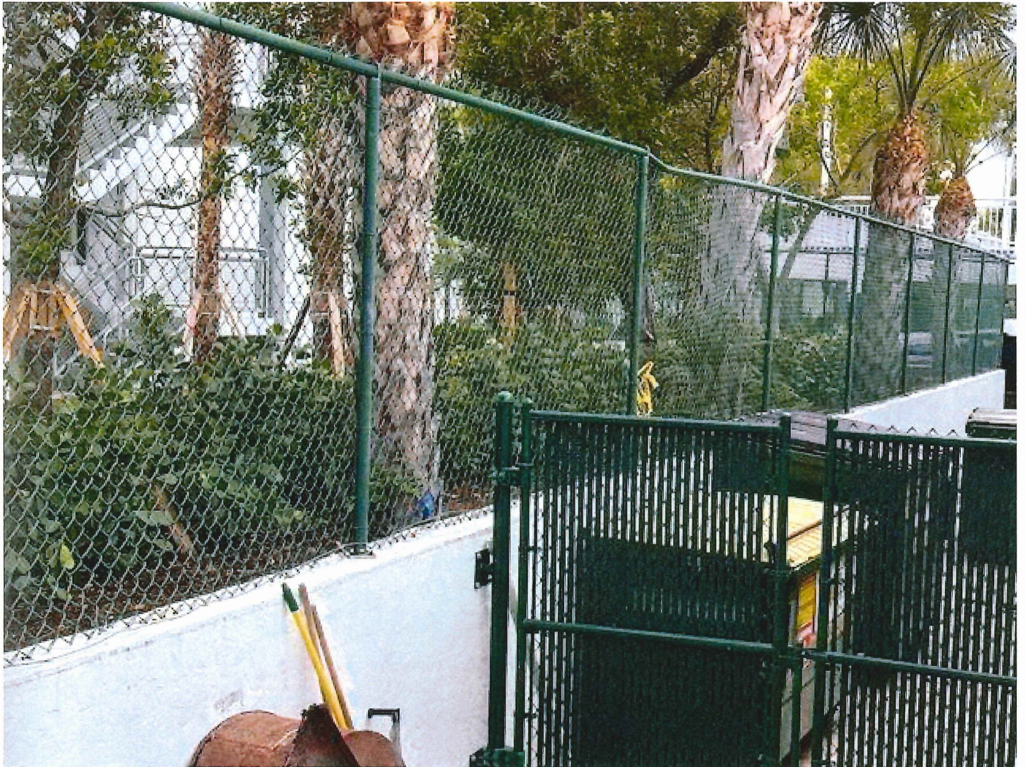
View from the south side of the Adjacent Property's parking garage wall and fence structure
