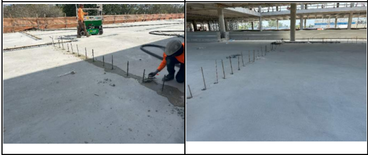
Figure 25. Photographs from Threshold Inspection Report No. 109 showing dowels extending through cored holes in slab. These dowels appear to be from the CMU wall below
