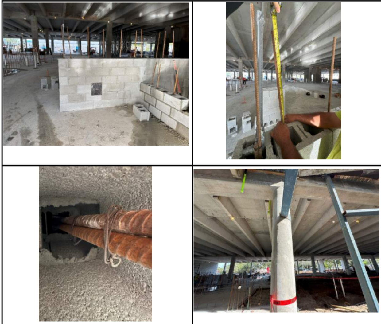
Figure 18. Photographs from Threshold Inspection Report No. 084. Upper photographs and lower right photograph appear to be of the first story prior to full installation of CMU walls. Note the lack of shoring indicating that the CMU walls were not constructed as bearing walls
