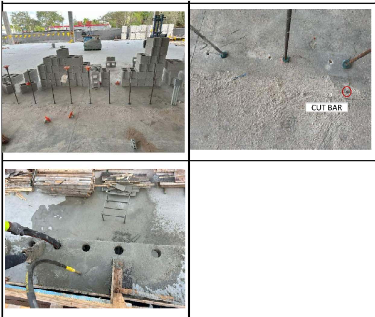
Figure 16. Photographs from Threshold Inspection Report No. 073 showing bars doweled 3 inches into slab-on-ground after original bars were mislocated (top photographs), and filling of grouted cells (bottom photograph)
