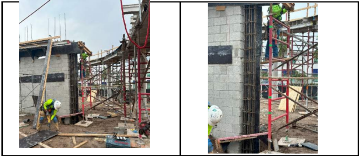
Figure 23. Photographs from Threshold Inspection Report No. 105 showing CMU wall in Area E under construction. Since the wall is being constructed prior to the roof structure, this CMU wall will take load from the roof structure as a bearing wall
