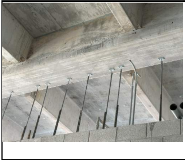
Figure 27. Photograph from Threshold Inspection Report No. 125 showing PTA connectors at bottom of soffit beam with the two screws attaching the plate of the anchor to the soffit beam
