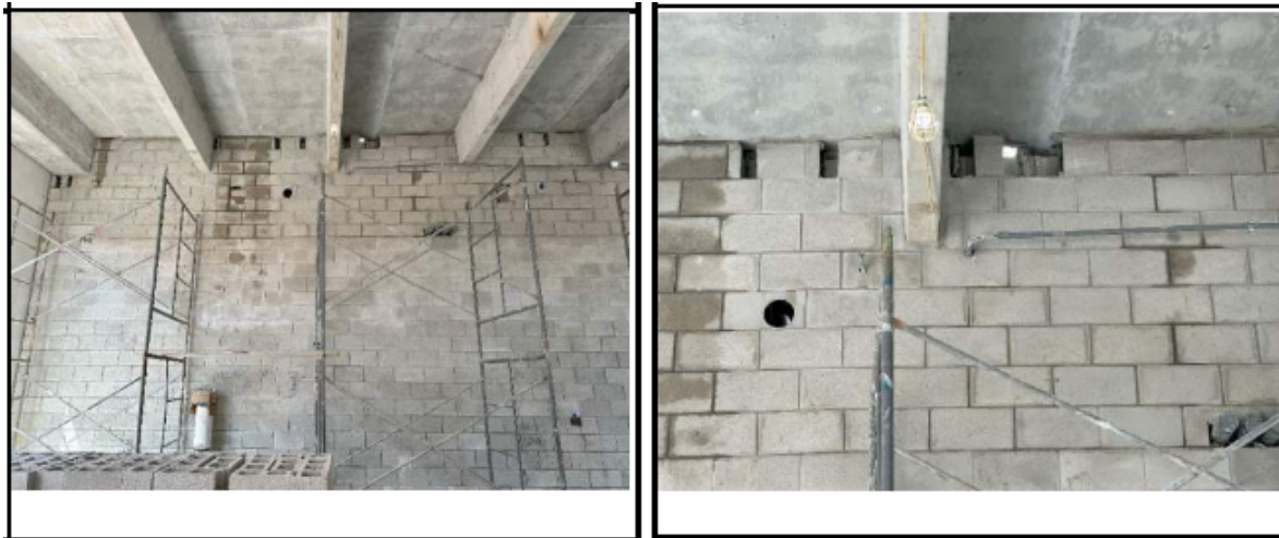
Figure 28. Photographs from Threshold Inspection Report No. 131 showing a wall that is nearly complete
