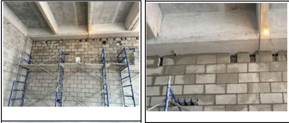
Figure 29. Photographs from Threshold Inspection Report No. 133 showing CMU wall at Level 1, Area D
