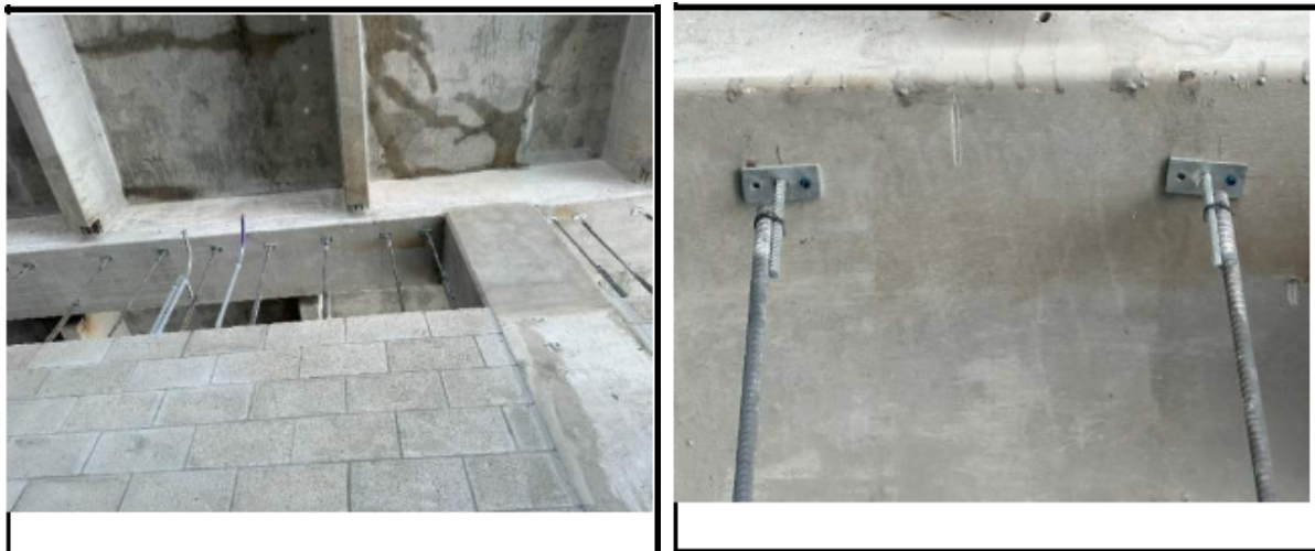
Figure 26. Photographs from Threshold Inspection Report No. 123 showing PTA connectors at bottom of soffit beam with only one screw attaching the plate of the anchor to the soffit beam
