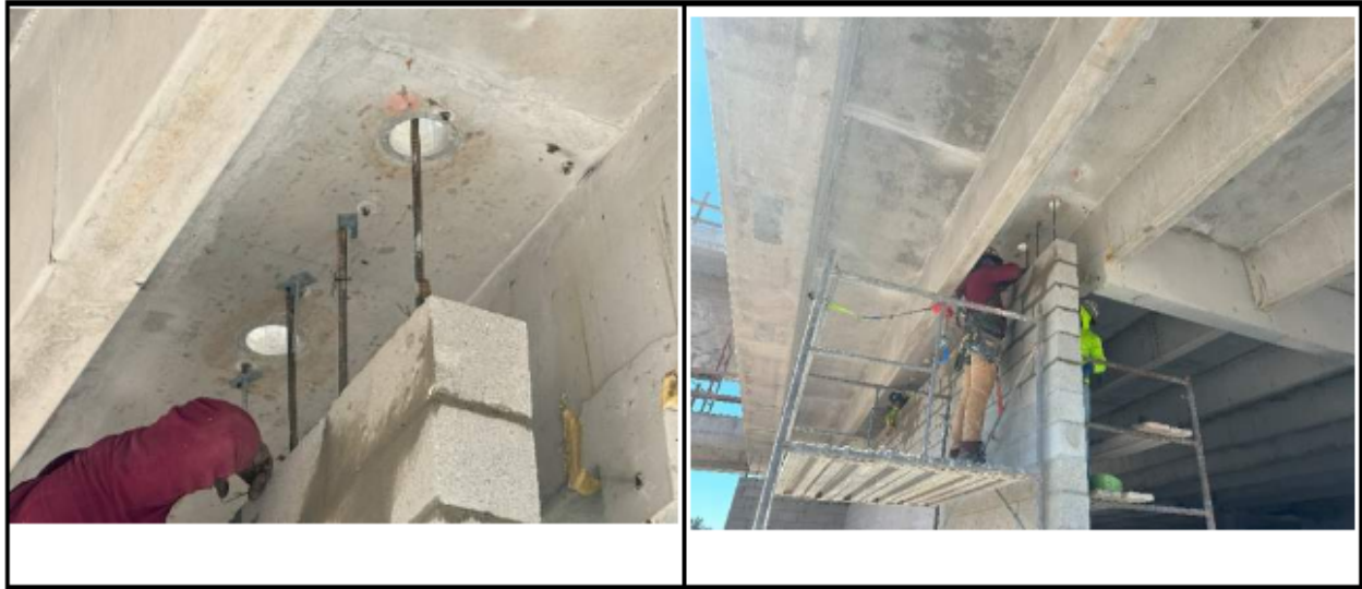
Figure 20. Photographs from Threshold Inspection Report No. 099 showing issue noted by inspector at top of “HQ Level 3 South CMU wall”. Note PTA anchors and connection of vertical masonry bars to above slab in left image. Note that the bars are generally spliced to anchors attached to the slab with screws
