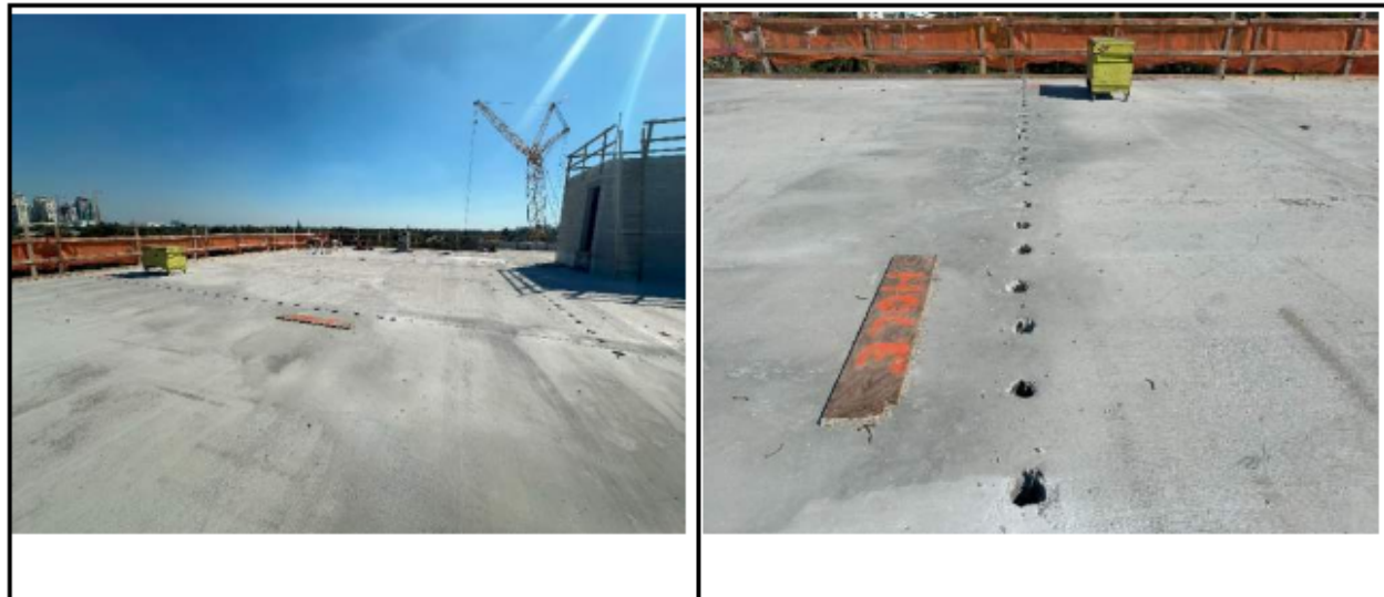
Figure 21. Photographs from Threshold Inspection Report No. 101. While not clearly stated in the report, these images are believed to be of the third floor slab
