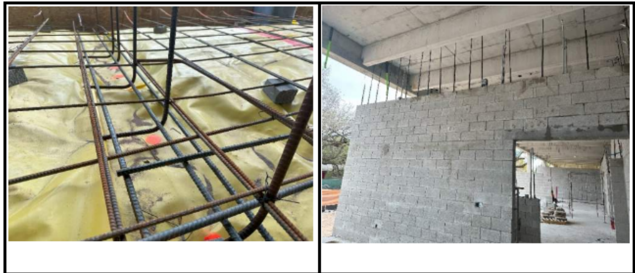
Figure 24. Photographs from Threshold Inspection Report No. 107. The photograph on the left shows hooked dowels at a thickened slab location under a wall. The inspector noted that the dowels needed to be shifted downwards. The photograph on the right shows a CMU wall in the first story under construction. Note that no shoring of the structure above is present, indicating that the CMU wall was not constructed as a bearing wall
