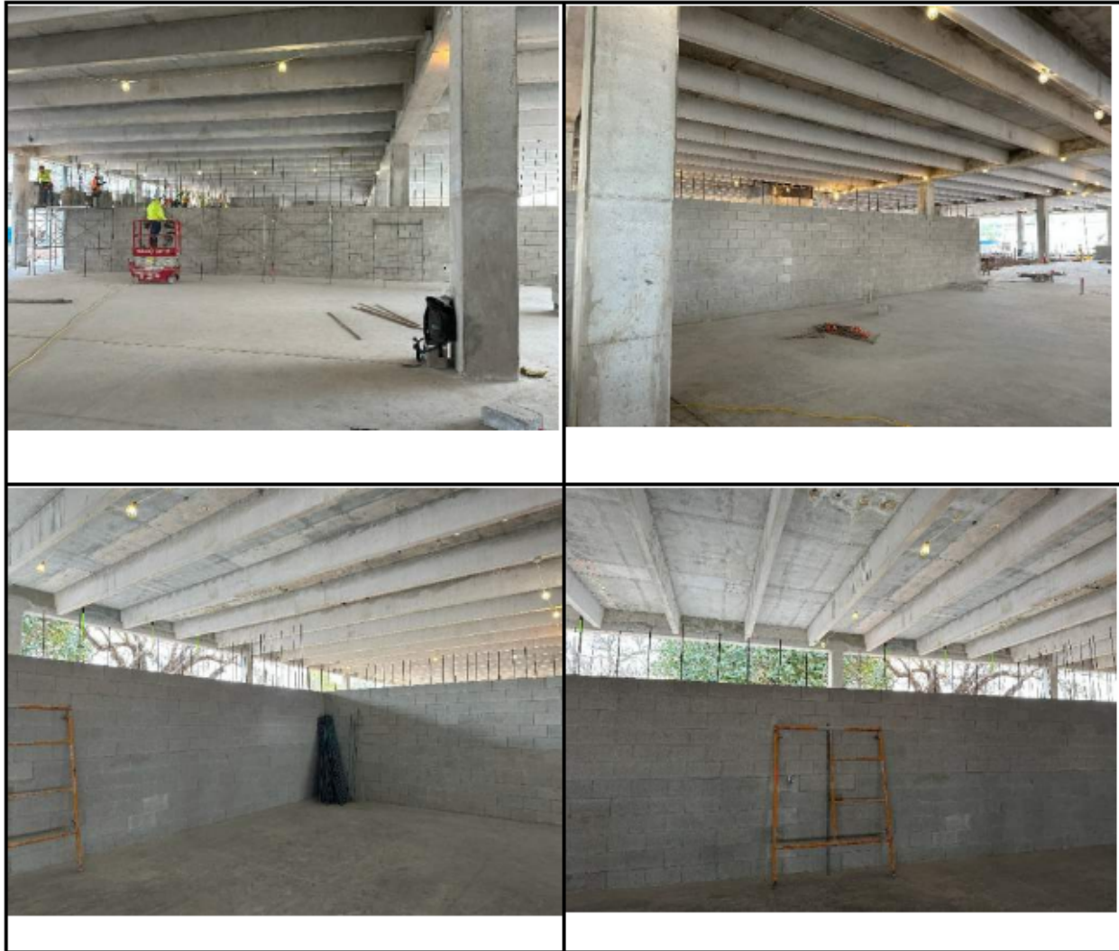
Figure 22. Photographs from Threshold Inspection Report No. 103 showing first story CMU walls under construction. Note the lack of shoring indicating that the CMU walls were not constructed as bearing walls
