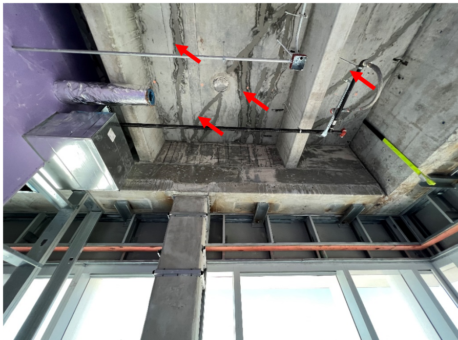
Figure 33. Example of cracks (see red arrows) in the reinforced concrete slab (at the roof) which have been repaired
