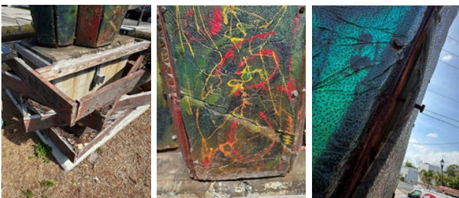
NE 13 Street Beacon showing fabrication issues.
