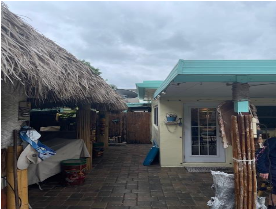
This is the west side of the chickee hut. This faces south
