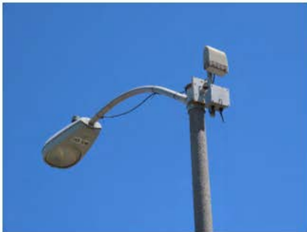
Shot Spotter technology installed on a streetlight
