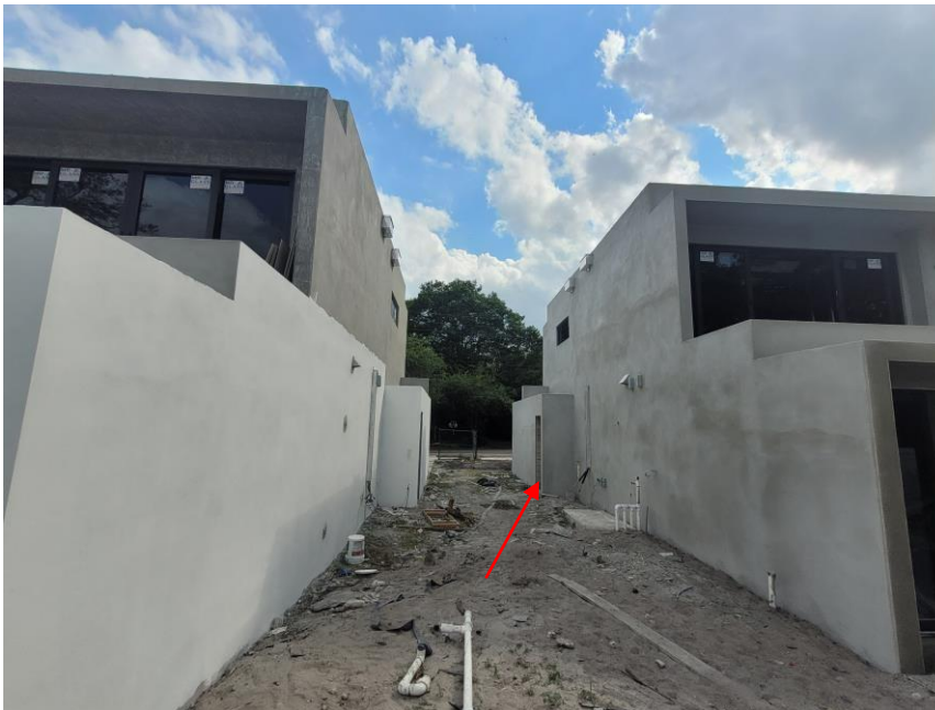
2935 and 2931 Riverland viewed from rear yard, 2935 Riverland is on the right. Arrow points to portion that projects into required yard.
