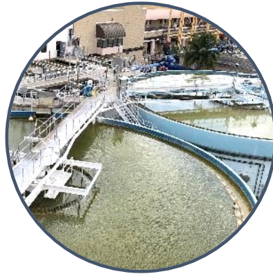
Fiveash WTP Lime Softening Constructed 1954*
