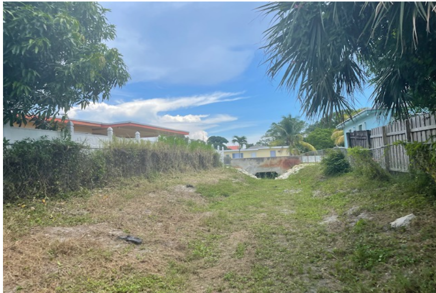
Figure 4: Grass and Weeds Growing between the Chain Link Fence Facing the Ditch and a Second Fence Facing the Private Property
