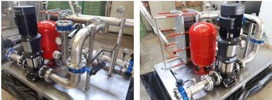
typical close loop cooling system skid
