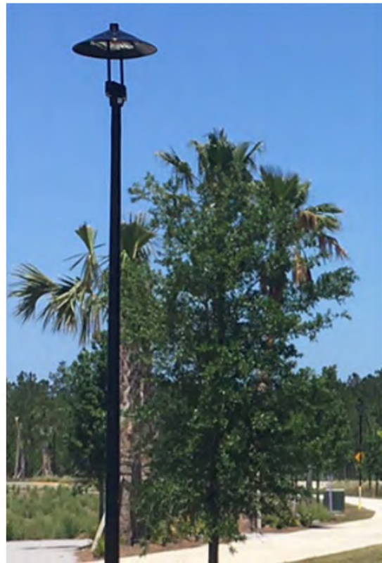
EPTC FIXTURE WITH TAPERED BLACK CONCRETE POLE
