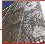
ARTICULATED METAL SCREENS
