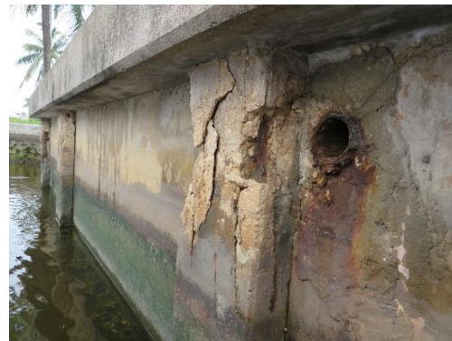
Figure 2.7.4 T-Pile Spall and Panel Cracking
