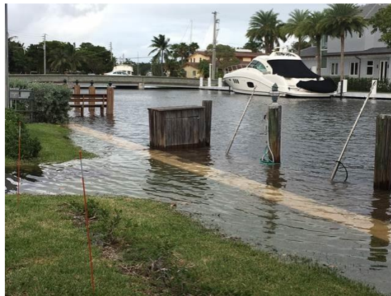
Figure 2.7.5 Cordova Road (Seawall No. 29) During King Tide Conditions
